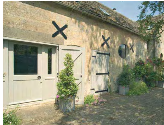
Figure 8.14: Retention of original features such as the stable joinery in this example is important to retain the character of the building
